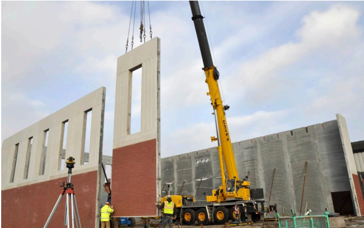
Fig. 1. Crane sets Precast Panels supplied by Wells Concrete with a Grove GMK5165-2 crane. Accessed on 29 January 2019 < https://cranemarket.com/blog/daves-crane-wrecker-service-sets-precast-panels-supplied-by-wells-concrete-with-a-grove-gmk5165-2-crane/ >
